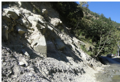
Fig. 8. Loose soil with boulders
