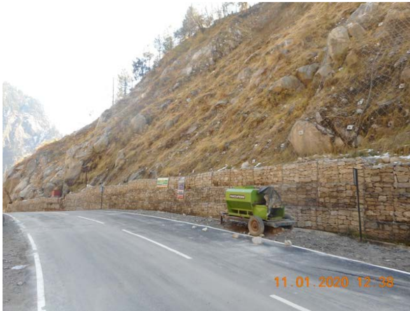
Fig. 19. Photograph showing the hill side rehabilitative measures (3-m high nailed gabion wall for toe stabilization and secured drapery system to secure large boulders adopted at site
