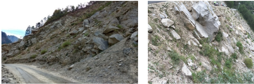
Fig. 3. Slopes adjoining the highway at Govindghat with boulder-soil matrix. The photo on the left shows strata above road level and the one on the right shows the strata below road level
