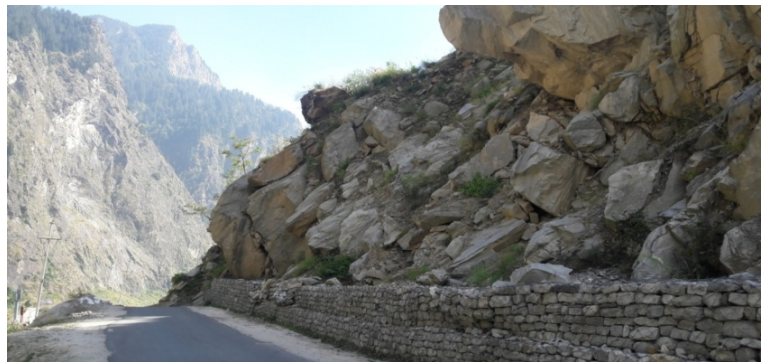
Fig. 7. Stretch with large boulders and open pores. Note the damage to the non-engineered handmade gabion wall
