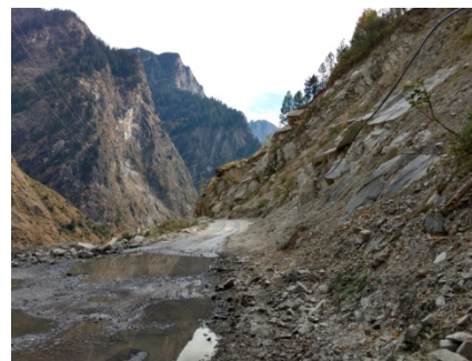
Fig. 9. Water and debris accumulated on road
